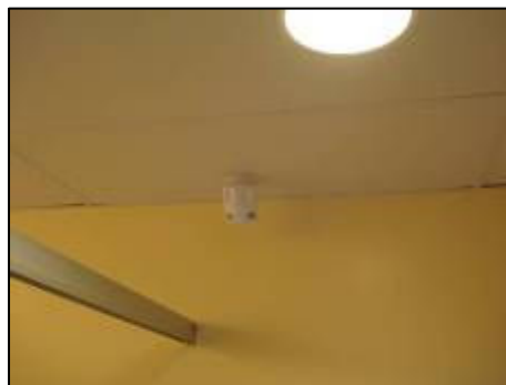
Audits include noting rooms that have light sensors, such as the one to the left.
