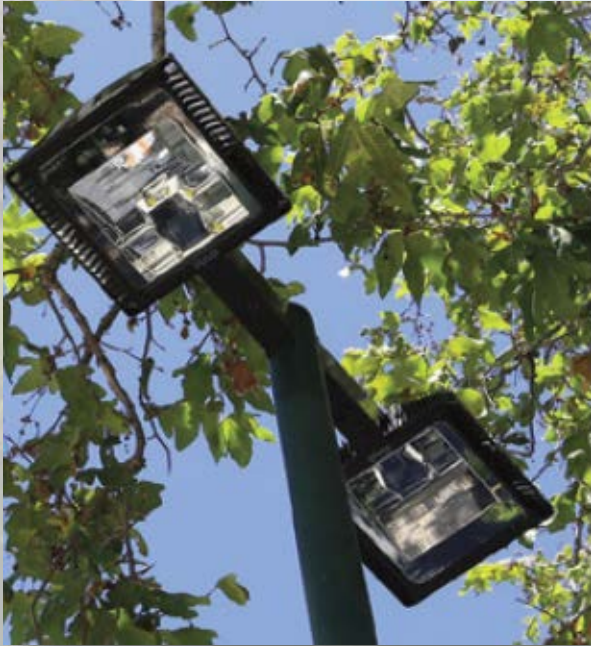
LED lighting installations throughout District parking lot save energy
