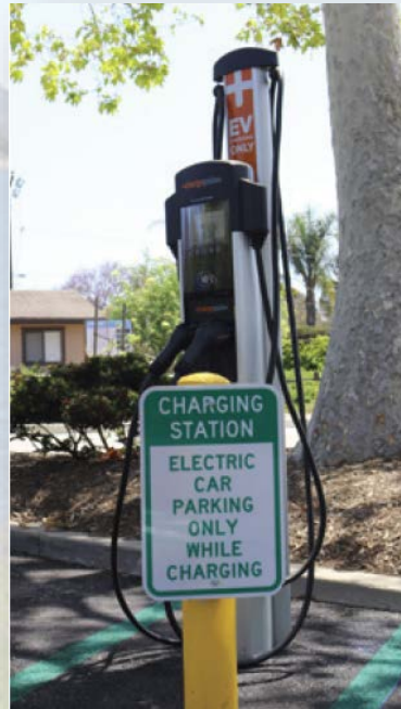
Vehicle charging station installed for employee and public use
